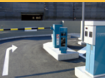
Parking Control System
