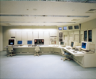
Fire Monitoring Panels in Control Center
