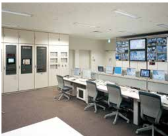
Fire Monitoring Panels in Control Center
