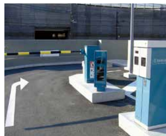
Parking Lot Driving Lane Control Systems
