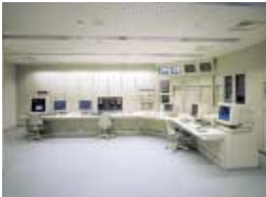
Fire Monitoring Panels in Control Center
