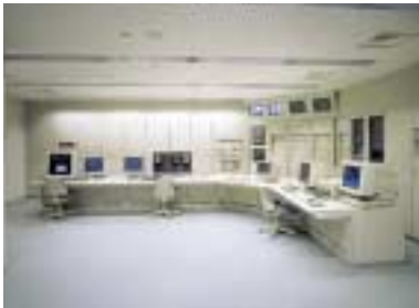
Fire Monitoring Panels in Control Center
