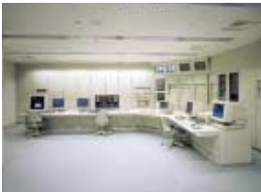
Fire Monitoring Panels in Control Center
